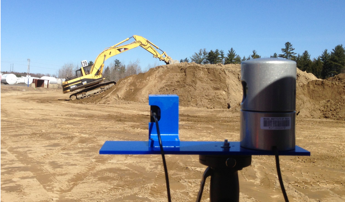
Figure 3-39: We captured operation of an excavator with a PointGrey camera (mounted left) and 3D LIDAR (mounted right).
