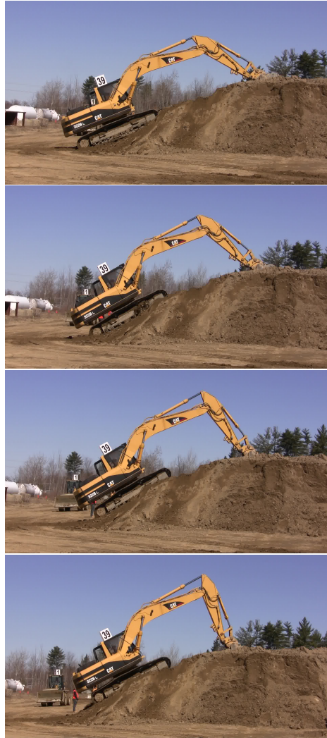
Figure 3-45: The excavator climbs the hill by sinking the bucket into the ground and pulling itself up.
